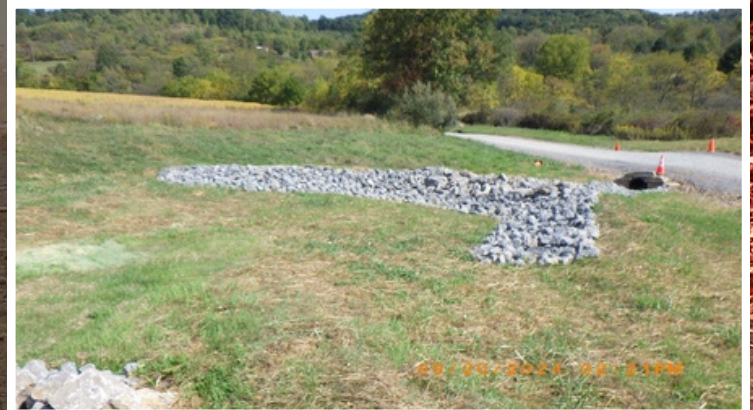
After: Top photo - Added underdrain outlet as well as crosspipe and 'through the bank pipe', both shown about halfway down the hill. Bottom photo- High volume of surface flow blew out project during construction. Once able to determine where the sources of the flow were, this berm was installed to help slow the water before taking it across the road and allowing it room to slow & infiltrate before reaching the stream.
